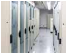
© 3U TELECOM GmbH
